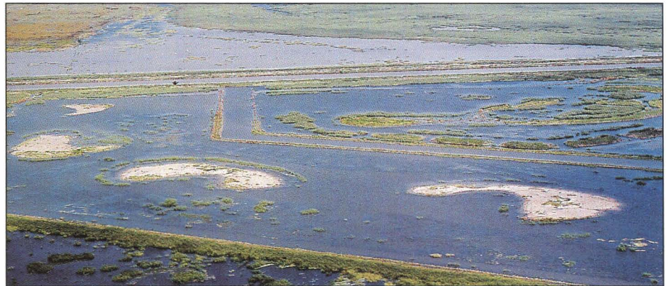
The nesting islands, pictured under construction at top, were built in Pool 5, an area that used to be the goose pen. Dikes allow water control separate from other pools.
